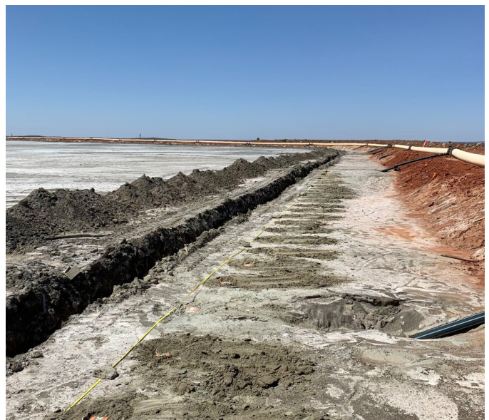
Fiber optic cables used on a mining project in Australia
