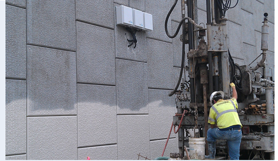
Geocomp field technician supervising the drilling of a borehole for the installation of an inclinometer. Note the iSite™ datalogger (for automated storing and transferring strain gage data) mounted on the MSE wall
