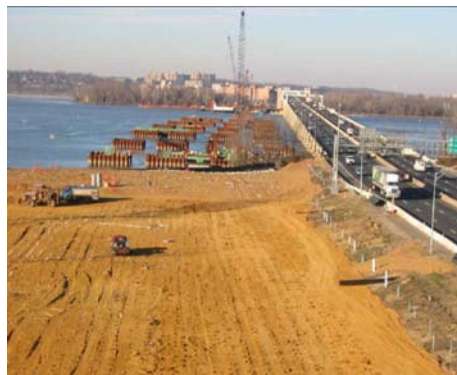
Pre-consolidation of soft foundation soils with earth surcharges and prefabricated vertical drains
